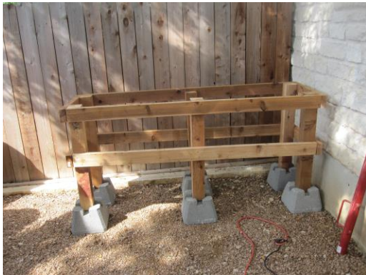
Figure 3 Frame in footing blocks. Note fence post driver to right of frame.
